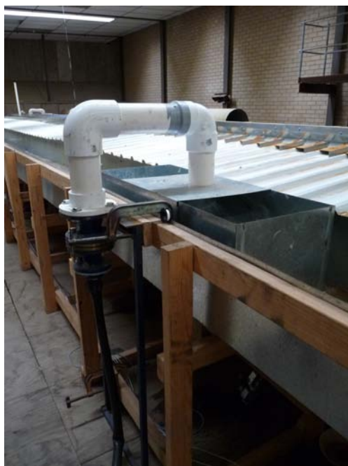
Figure 3. Flow Distribution Device Installed Above an Outlet
