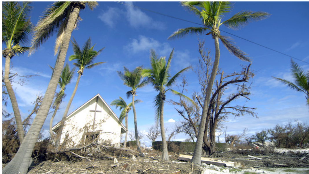
A damaged church, dead trees and debris on Wake Island left by Super Typhoon Ioke in 2006 (US Air Force photo/Tech. Sgt. Shane A. Cuomo)
